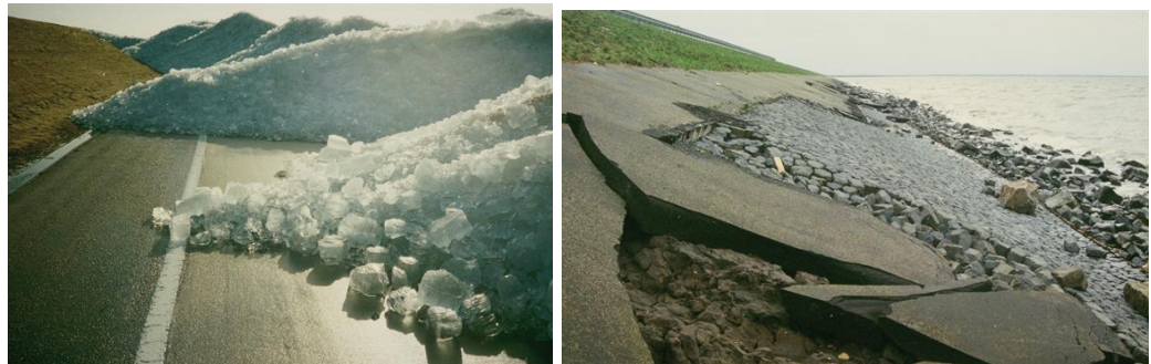
figure 21 Ice on the Houtribdike, Lake Marken 1987 and observed damage afterwards (Hans Johanson, Rijkswaterstaat DWW)
